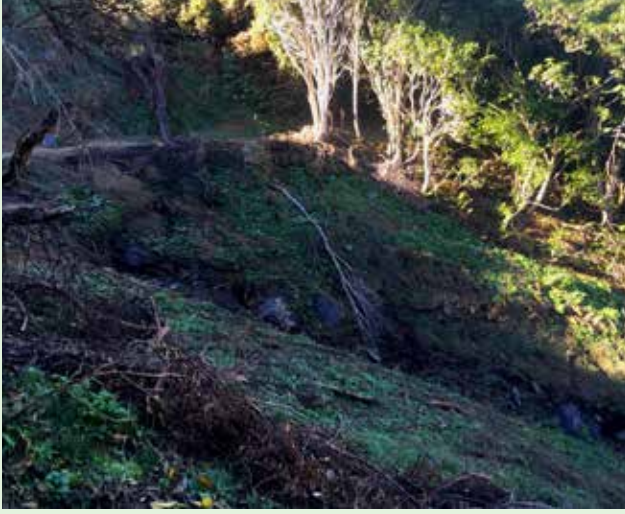
May 2022 - Looking across the landslide that had five months earlier gouged out this path, dissecting East Track in Hinewai. Photo credit: Alice Webster.
